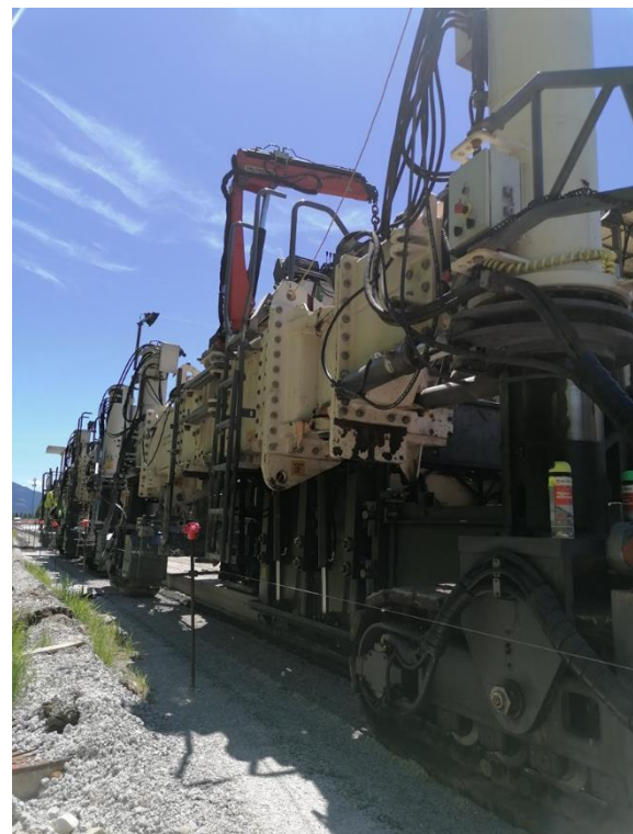
Figure 10. Concrete paver with even 12 crawler tracks for paving bottom and top concrete, Source: K. Hrapović, 2021
