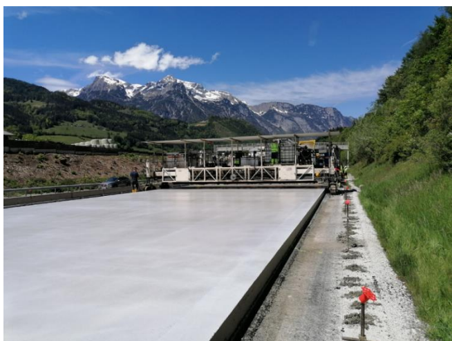
Figure 29. Finished, two-layer concrete pavement on the Austrian A10 Tauern motorway, Source: K. Hrapović, 2021
