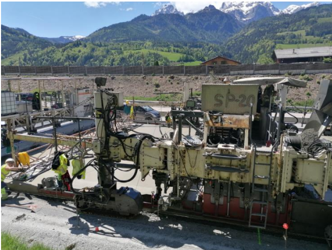
Figure 12. Concrete paver with even 12 crawler tracks for paving bottom and top concrete – middle part, Source: K. Hrapović, 2021
