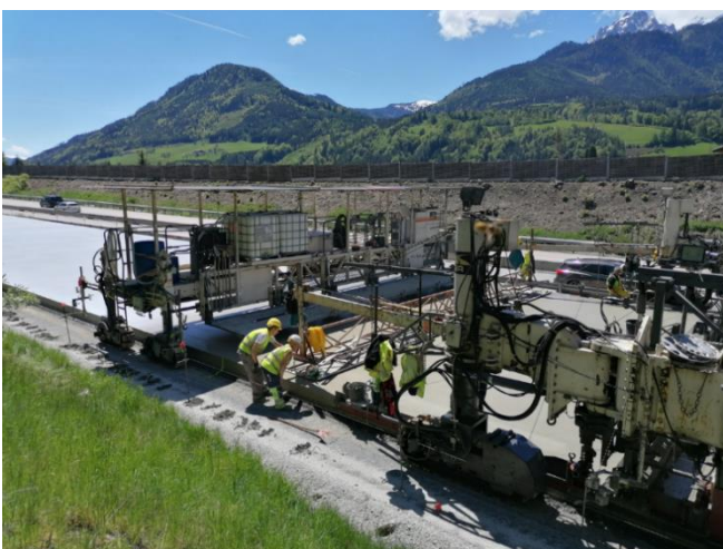
Figure 13. Concrete paver with even 12 crawler tracks for paving bottom and top concrete – back part, Source: K. Hrapović, 2021
