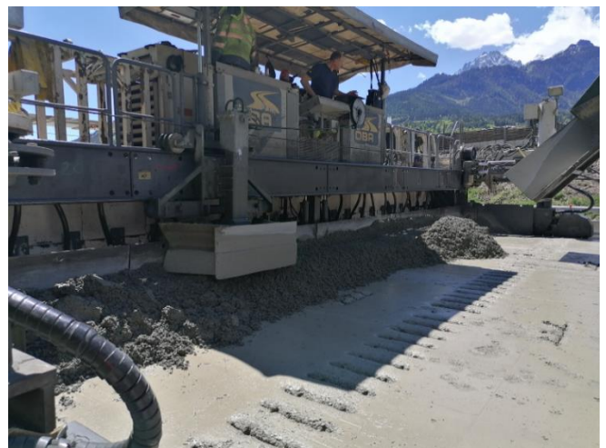
Figure 25. Installation of top concrete after automatic installation of dowels in the bottom concrete, Source: K. Hrapović, 2021
