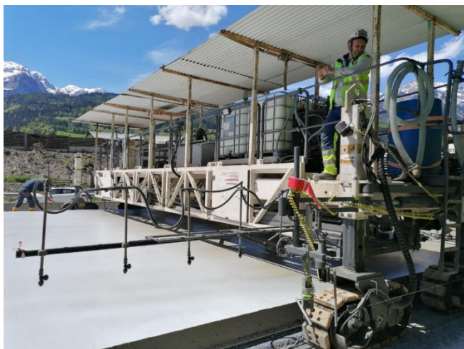
Figure 28. Application of the chemical surface protection over the finished concrete, Source: K. Hrapović, 2021
