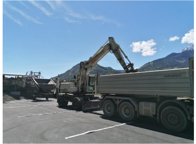
Figure 14. Loading the concrete from the truck by means of an excavator, Source: K. Hrapović, 2021
