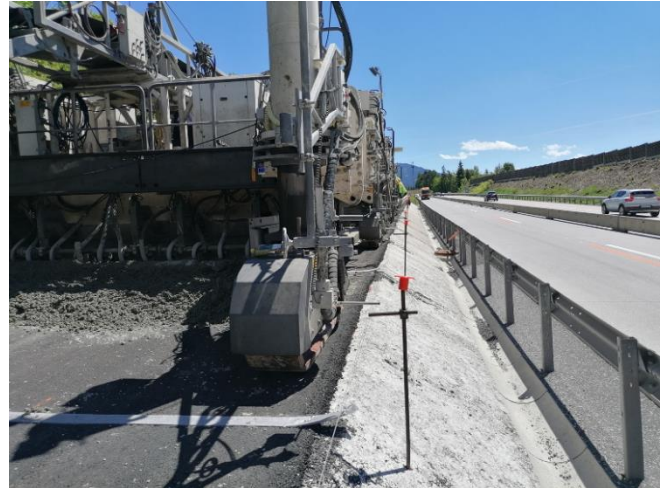
Figure 18. Flat drain laid on milled bituminous base under concrete pavement, Source: K. Hrapović, 2021
