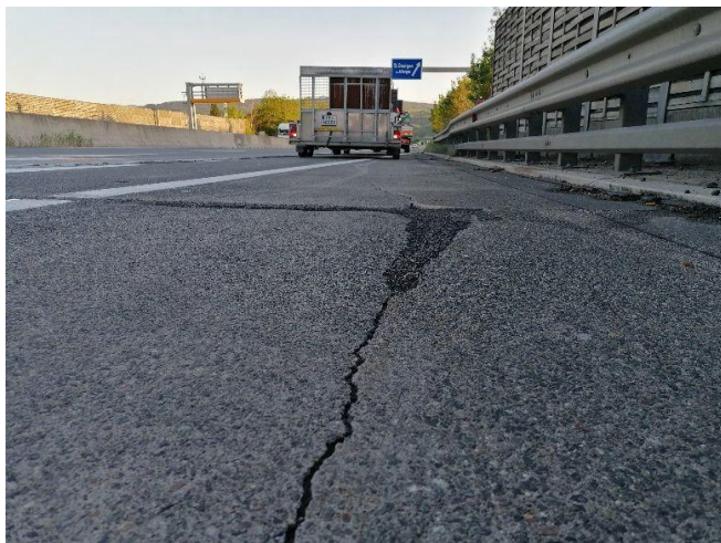
Figure 8. Cracks and damaged surface filled with cold asphalt Source: Author 2021
