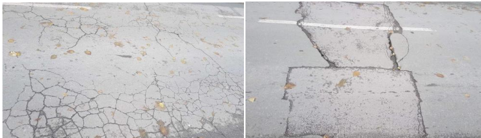
Figure 5. Dominant distresses in Miše Dimitrijevića street (left- alligator crackings, right- patchings)
