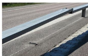
Rectangular steel lane dividing barrier (Photo - GEMS)
