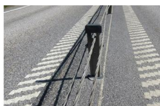
Wire rope lane dividing barrier (Photo -GEMS)
